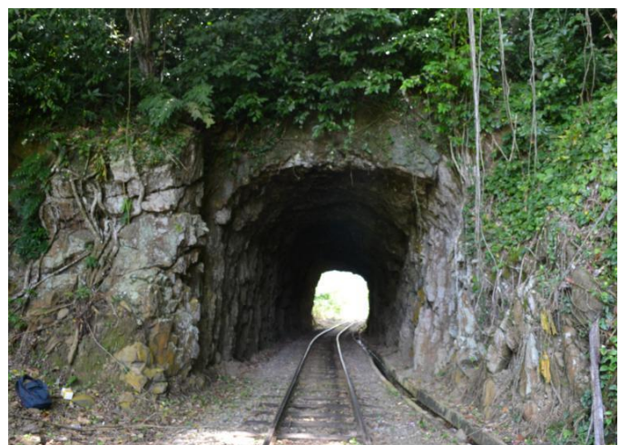
Photo 1: Entrance of Tenom Tunnel. Photo direction – east southeast (ESE) to west northwest (WNW)
