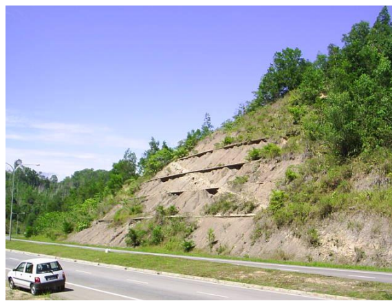
Figure 8: The cutting of hill slope, removing trees and vegetation from the hill slope reduces the stability of the slope (Location: Highway Batu Sapi - Sibuga)
