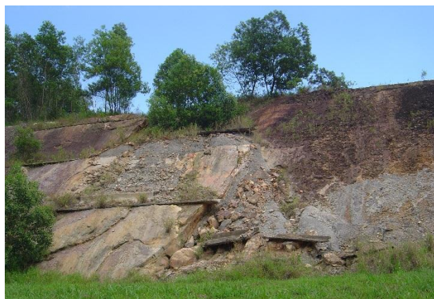
Figure 7: Dangerous slope failure near by the Indah Jaya
