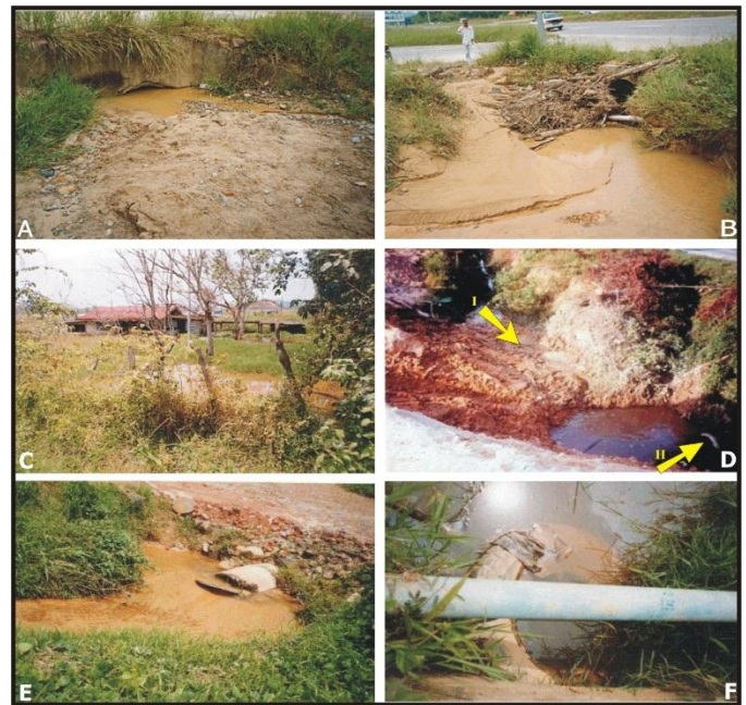
Figure 5: Factor causing environmental problem in the study area. A. Clog along the drain. Small and shallow ditch and siltation in the upper part of the culvert. B. Small culvert and partition of debris. C. Demolish house in the swampy area and grass field in the new natural sediment trap originated from paddy field. D. Congestion at the channel flow. The '90° corner' drainage channel (arrow I flowing to north and arrow II to the west) and small culvert (arrow II). E. Improper monitoring and maintenance of drainage channel to the solid waste and wild grass. F. Lack of enforcement of the environmental regulation (partition of debris and siltation).
