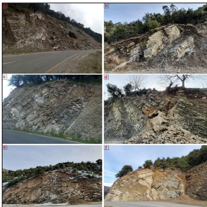
Figure 3: Field photographs of the investigated area; (a) Planar failure condition, here foliation plane dipping towards the road at zone Z3A; (b) foliation plane dipping towards the slope and a set of vertical to sub-vertical joint intersection the rock mass at Z4D which is failed due to planar failure; (c) foliation plane dipping towards slope at >45° angle and an inclined valley dipping joint intersecting the exposure that is giving the birth to topple failure at Z5E location; (d) field photograph is showing wedge failure condition between joints set1, set2, and bedding plane at Z2A location; (e) a planar failure condition due to joint set1 and set2 in which both are dipping in the same direction of slope which cause planner failure which is already failed at Z6A location; (f): a wedge failure condition due to joint set2 and set3 which is already failed at Z5G location.
