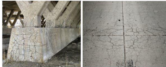
Figure 1: Cracks formed in concrete due to ASR (Mercan, 2018)
