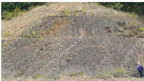
Photograph 4: Rock cut slope for slope B. Interlayer of sandstone and shale with similar amount (Photograph orientation N 182°).
